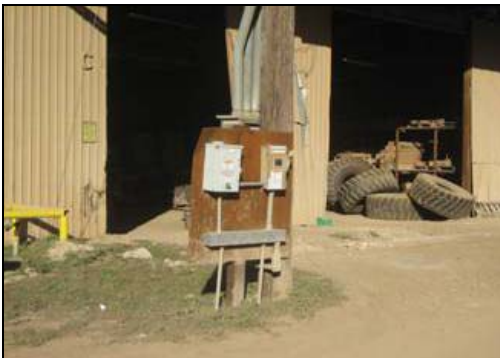
Electrical Equipment Exposed
